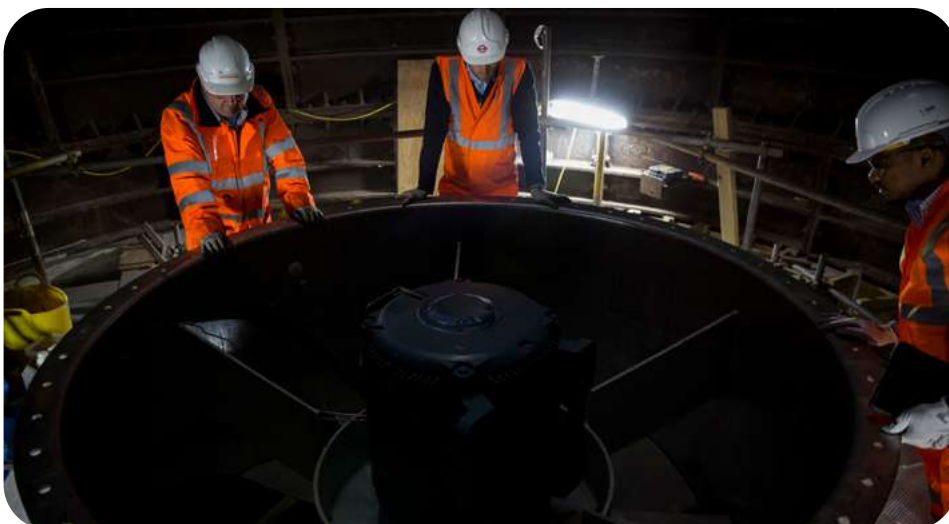
→ Construction of the Bunhill 2 Energy Centre, which re-uses waste heat from the London Underground to heat homes © Joel Ford/TfL
